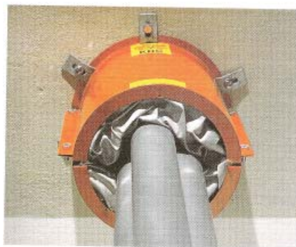
Pipe bundle in KBS Pipe Seal M
